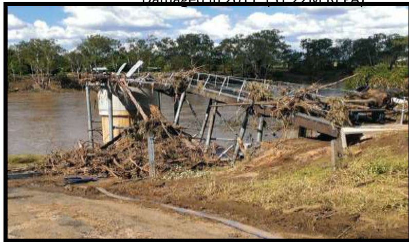
Re-damaged in 2013 ($2.6M REPA)
