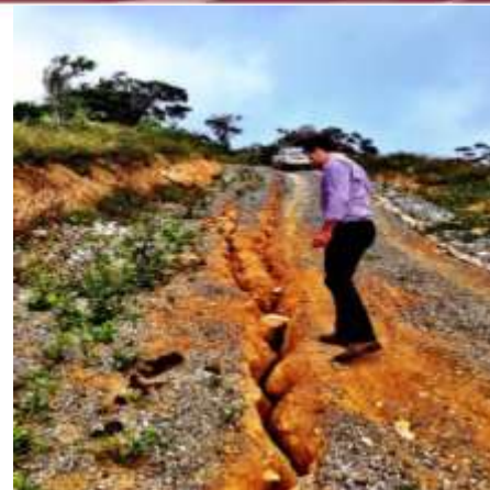
Repeated damage in 2010, 2012 and 2013
