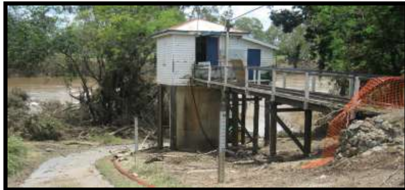
Damaged in 2011 ($1.22M REPA)
